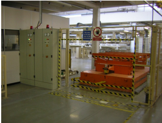
AGV at charging station – opportunity charge
