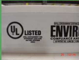
Spill Containment Barrier
